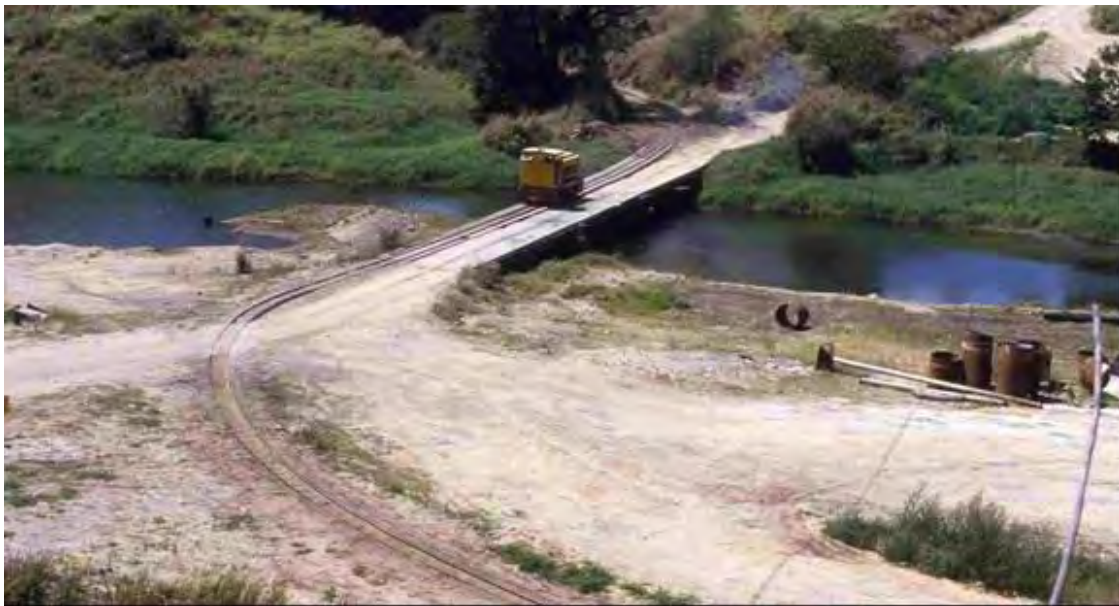
The original dual purpose timber low level road/tramway bridge over the Pioneer River at Mia Mia. A MRC sketch of the existing bridge on the next page shows the tramway is on a rising grade and curve compared to the attached road bridge.
