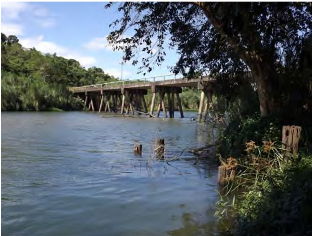
Mulgrave River Bridge built in 1980. Concrete piles and headstocks with prestressed concrete deck units. Rails set flush with the asphalt deck wearing surface. Some remnants of the previous timber bridge remain beside this bridge.
