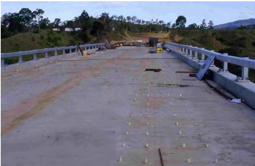
Construction of cast-in-situ concrete deck on prestressed girders showing location for installation of tram rails.
