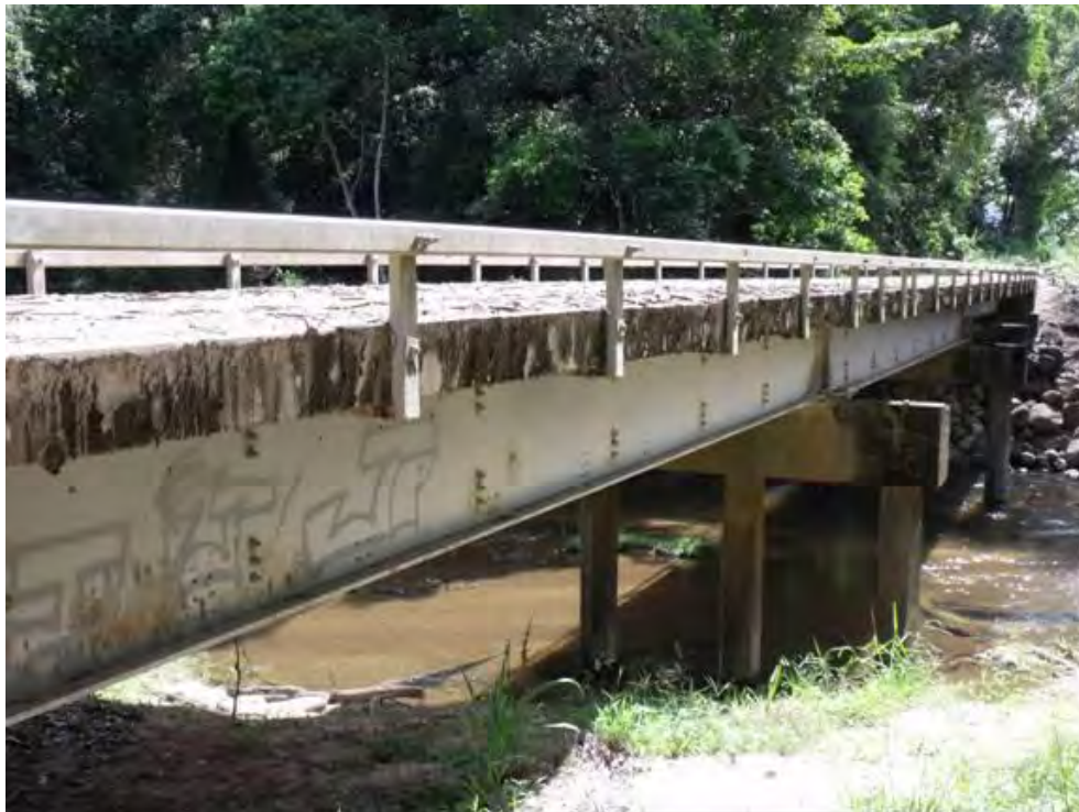
Concrete piles and headstocks support steel girders and concrete deck. The rails are cast into the concrete deck and finish flush with the top of the deck.
