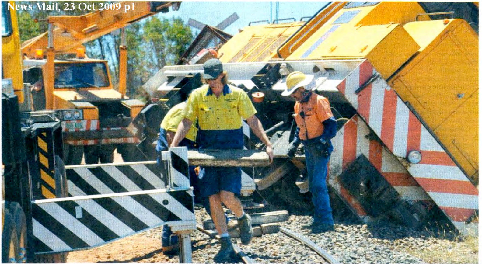
Heavy lifting was required to put this loco back on track after a derailment near Nedwich Road, Alloway, yesterday.
