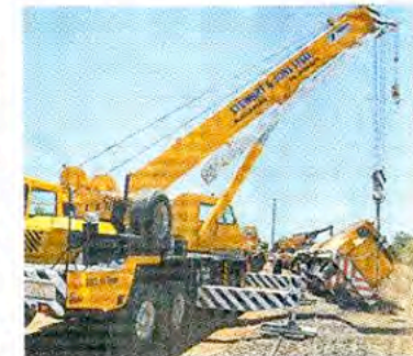
Heavy cranes were brought in to help lift a derailed loco back on track near Nedwich Road yesterday.
