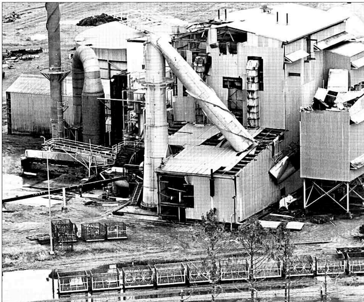
Cane-enabled: The Mourilyan sugar plant, south of Innisfail, was damaged by Cyclone Larry
