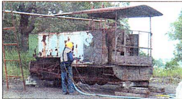
Amazing what a bit of sandblasting and a coat of paint can do. Old Number 4 being prepared for a repaint during a Rotary working bee.
