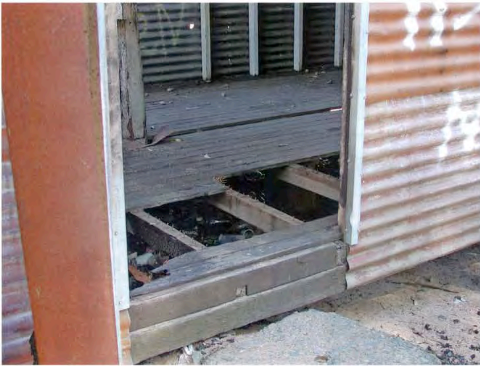
LEFT: Interior showing floor construction, from the back door. There appear to be three timber beams set on the stumps and running the length of the building, with a conventional floor joist and header construction under the floor boards. Note that the header and joists are notched and interlock to prevent twisting.
