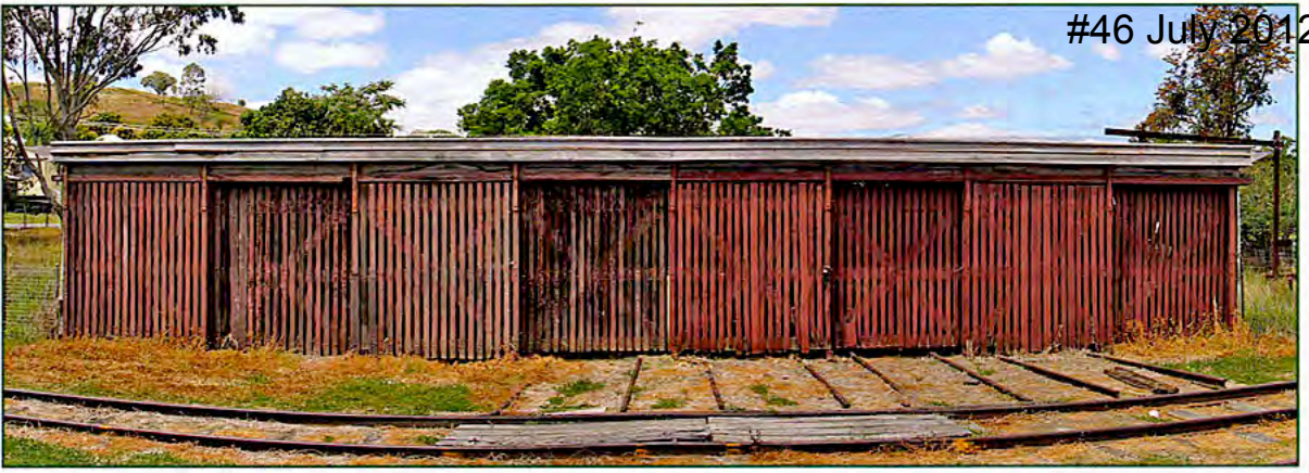
ABOVE: This view has been created by stitching several shots of the shed together to make a panorama. Note that only four stalls have 3' 6" gauge tracks leading to them, and that only two of these have timbers between the rails to make it easier to move the section cars and trailers to and from the main line. All of the shots were taken from the same position, thus the seemingly curved track. In reality the track is fairly straight at this point.
