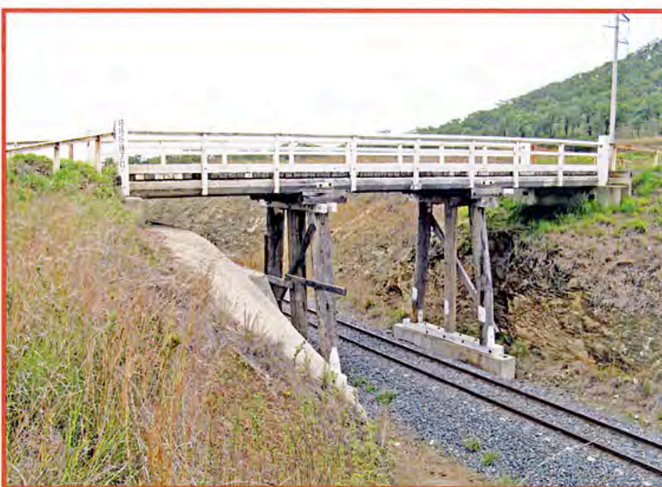
ABOVE: Side view of the QR overbridge near The Caves, Central Queensland, 2007. Note the fairly new appearing concrete footings: it is quite possible that bridge pilings would originally have been driven into the ground, rather than sitting on a pier.
