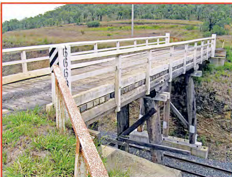
BELOW: Three-quarter view of the QR overbridge near The Caves, Central Queensland, 2007. The steel railing in the foreground is meant to discourage anyone climbing down the cutting. The extra length horizontal brace and short diagonal brace are likely the result of a repair at some time, rather than design.
