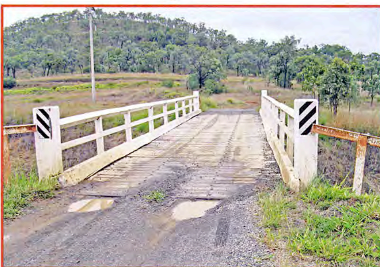
QR overbridge near The Caves, Central Queensland provides single lane access to a rural property from the Bruce Highway. The bridge deck and railings seem to be in good repair; note that the top railing (likely a 6 x 6) is square and angled with a corner upwards for weather protection, 2007.
